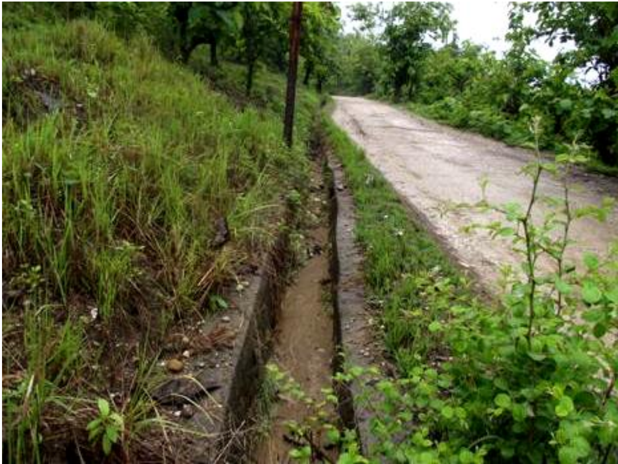
Plate 7-47 Beaco and Viqueque road condition
