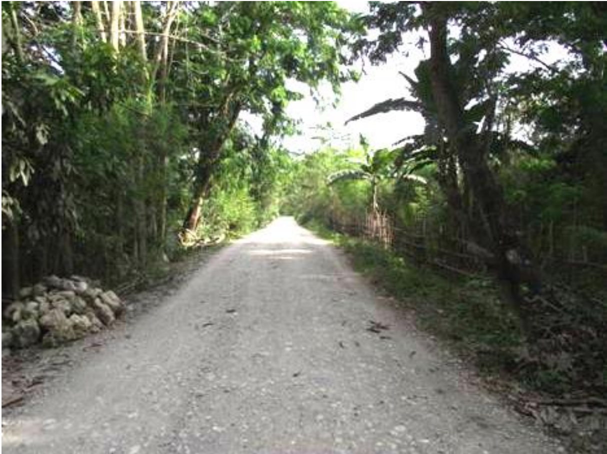
Plate 7-46 Beaco and Viqueque road condition
