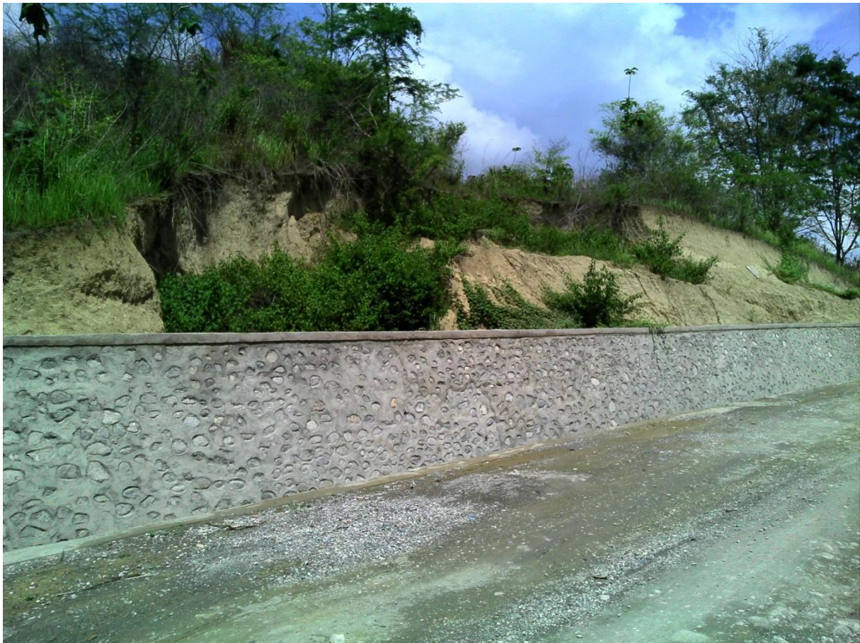
Plate 6-41 Slope failure at Nova Betano West behind a retaining wall along the road to Same
