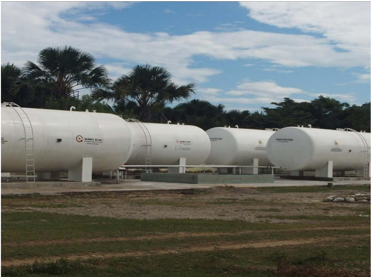
Plate 6-49 Oil storage tanks at Tibar
