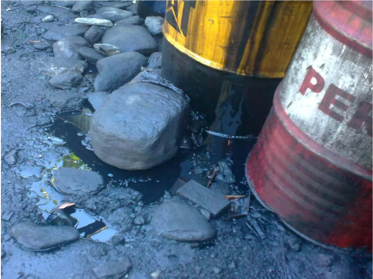
Plate 6-48 Typical leaking oil drum
