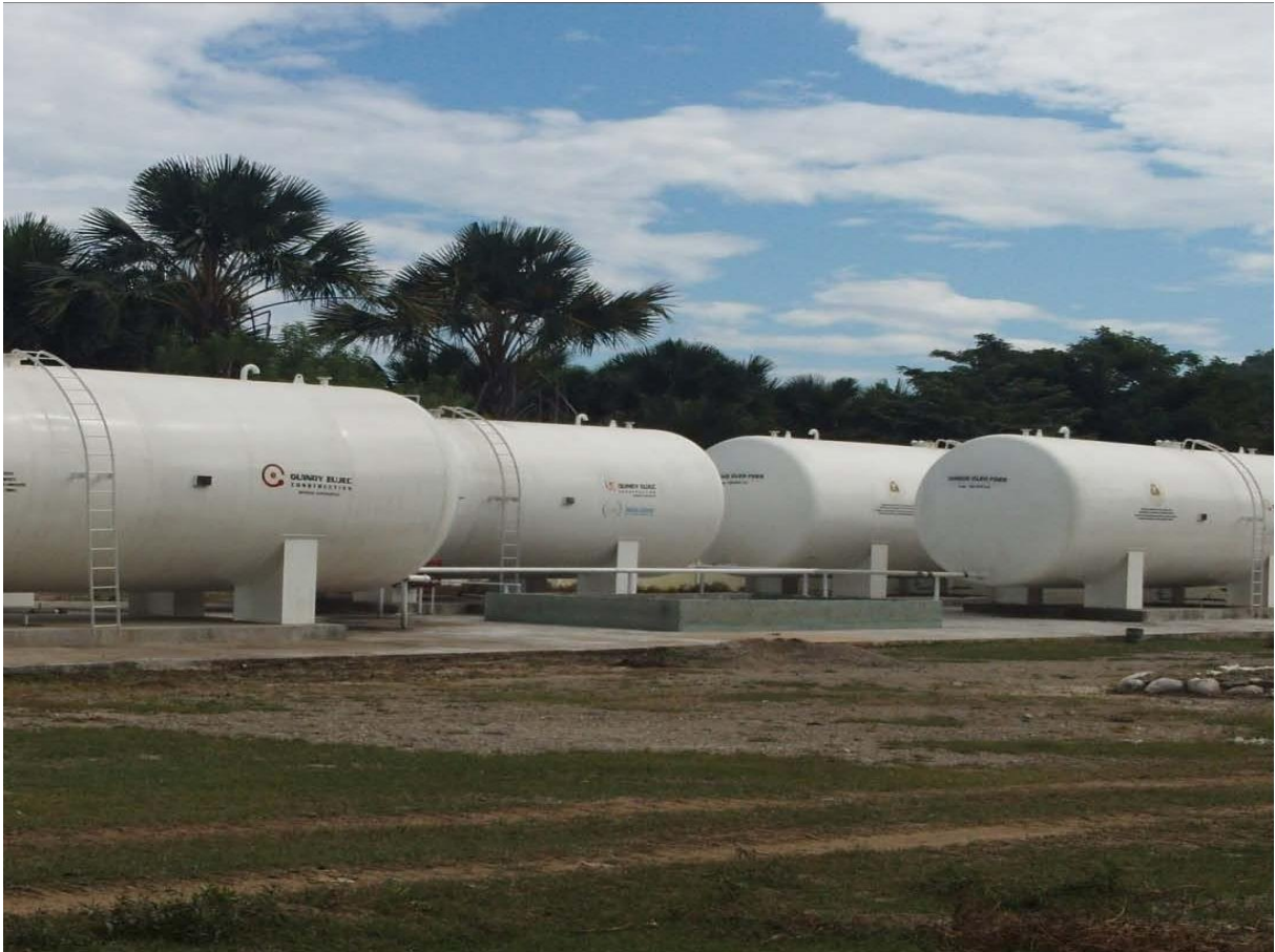
Plate 17-2 Oil storage tanks at Tibar
