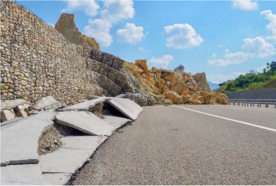
PHOTO: The freeway has been blocked by a landslide for months. (ABC News: Michael Barnett)
