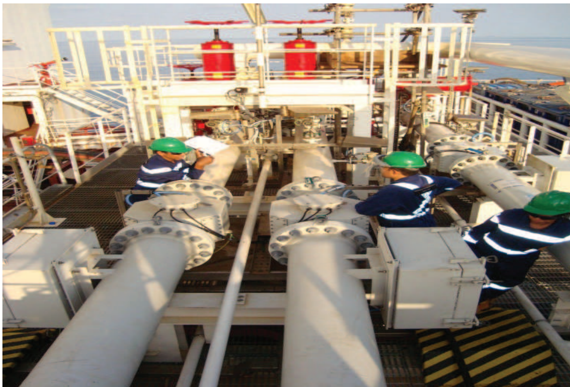
Picture 10: Metering Audit on the Kitan GD FPSO Facility
