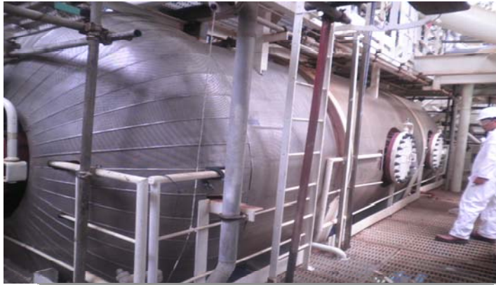
Figure 24 ANP's Inspection on Wet Commissioning System 505 FPSO GD in Singapore
