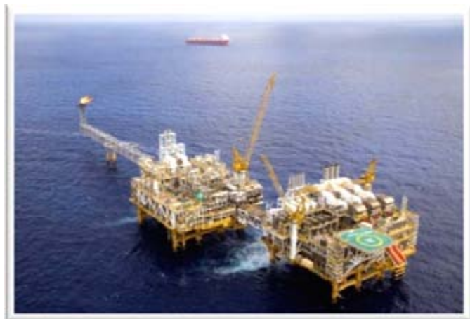
Figure 6: Bayu Undan Facility
