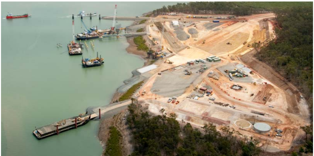
Aerial view of GLNG material offloading facility site on Curtis Island, 5 October 2011.
