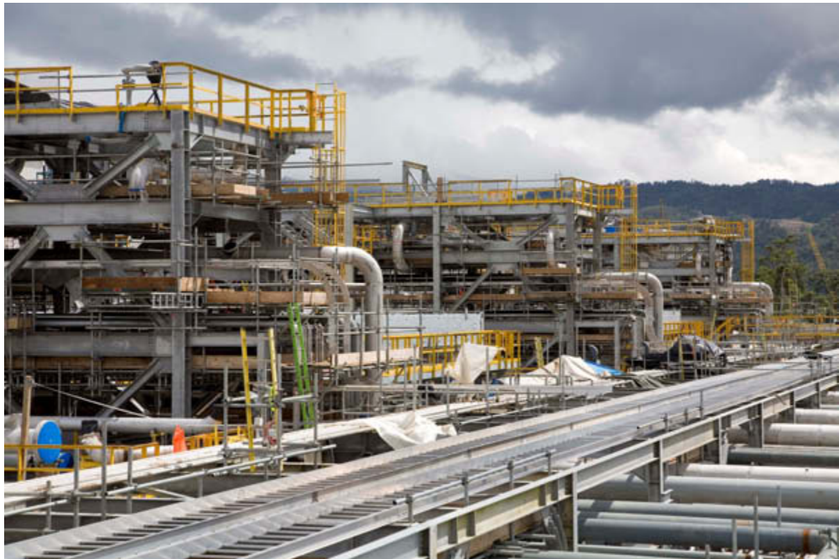
Hides Gas Conditioning Plant, June 2013.
