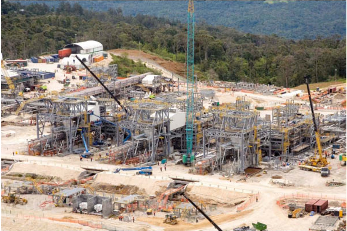
Hides Gas Conditioning Plant, May 2013.
